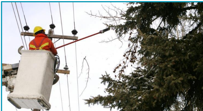
Image 4: Trees and powerlines don't mix well
