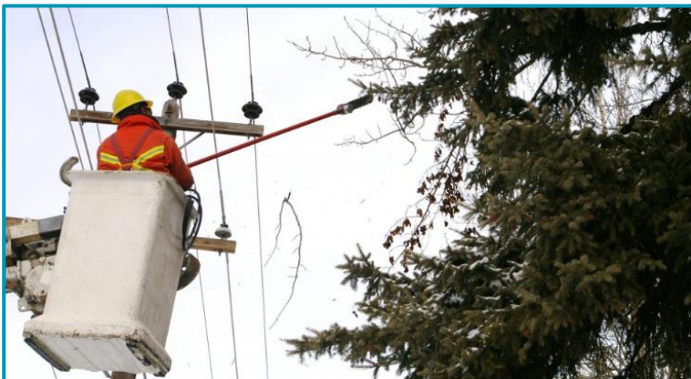
Image 4: Trees and powerlines don't mix well
