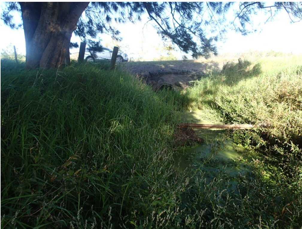
Photo 6. SH1 culvert outlet pool with pond weed in foreground transitioning to azolla. Pool divided by kikuyu covered fence wire at the boundary, partially obscuring culvert in background.
