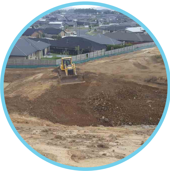
Guideline 1 Large scale earthworks wipe the slate clean but can disrupt and destroy the natural environment.
